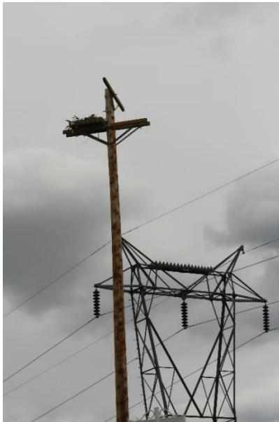
Transmission structure with nest deterrents installed. An osprey nest was successfully relocated from the structure and installed on the artificial nesting platform shown here.
