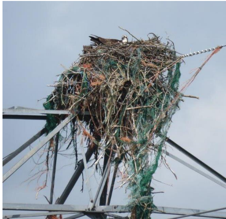
Example of a nest that has become a safety hazard. The nest is large and the material is contacting energized components of the structure which could lead to a power outage and even a nest fire.
