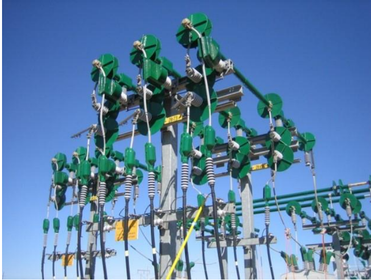
Substation with Greenjacket™ covers installed.
