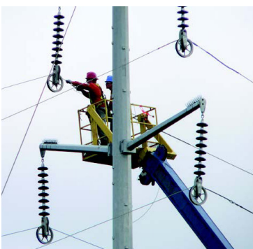
Above: Once structures are erected, transmission line wire, called conductor, can be strung.
