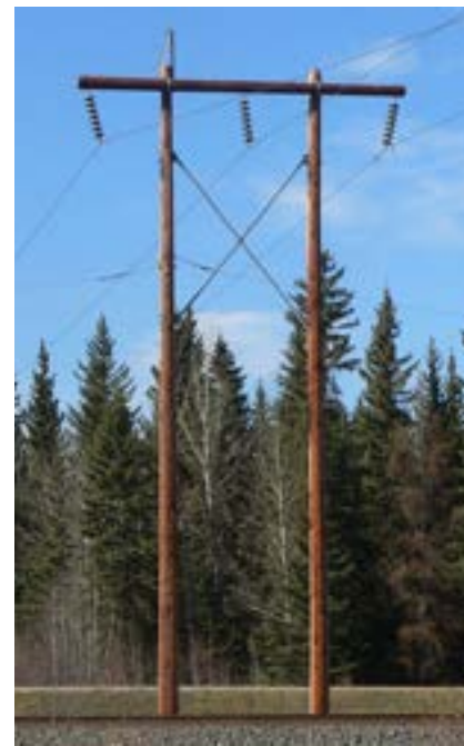
Above: These existing H-frame structure types will be replaced with structures that are similar in appearance and size.
