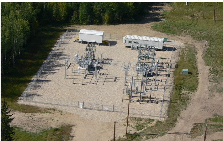
The new Berland River Substation will look similar to the photo above
