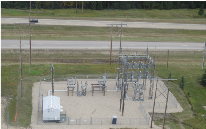
The existing Fox Creek Substation
