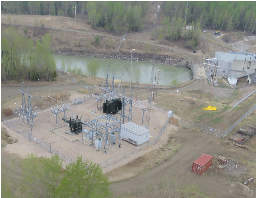
The existing Brazeau Outlet Works 2945 Substation.
