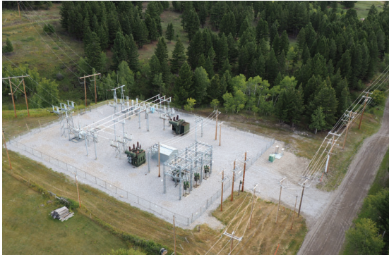
The existing Coleman Substation.
