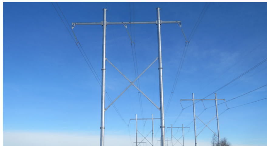
Above: Steel H-Frame structures on the new transmission lines will be between 26 to 32 metres tall.
