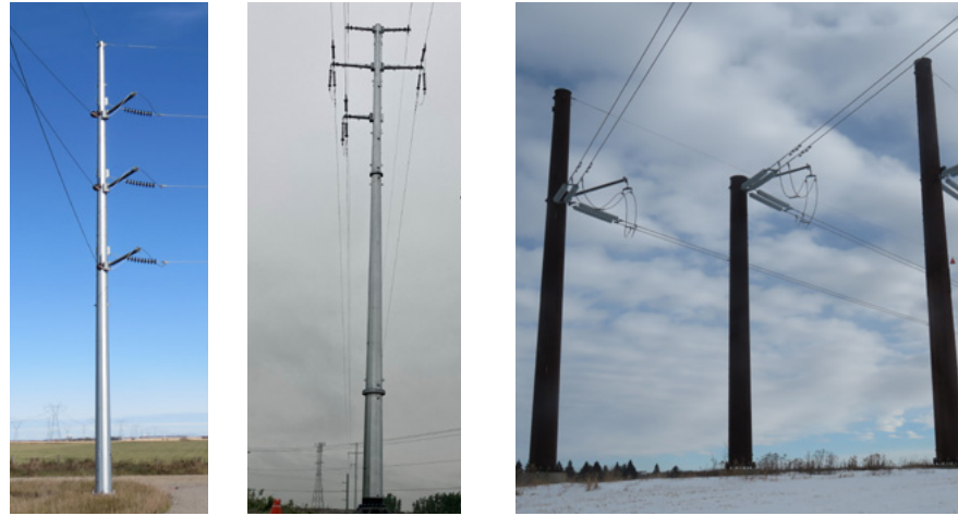
Above: Self-supporting steel poles will be used to anchor the ends or corners of the new transmission lines. These poles will be between 28 to 40 metres tall.
