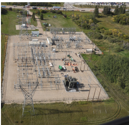
The North Calder Substation.
