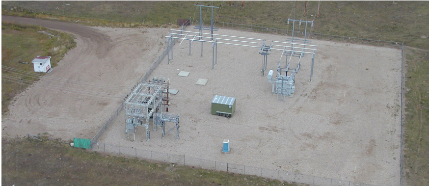
The existing Pigeon Lake Substation.
