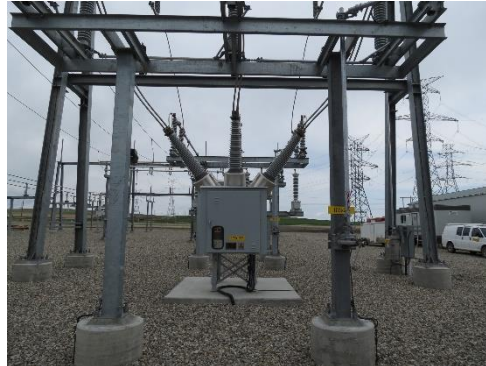
138 kV circuit breaker
