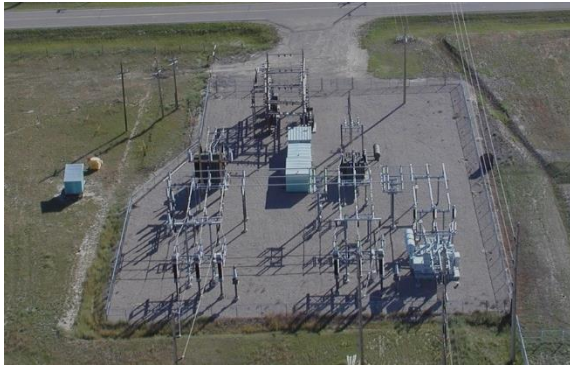
Empress 394S Substation
