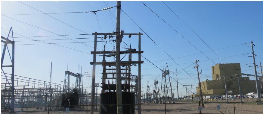
The existing Keephills Substation.
