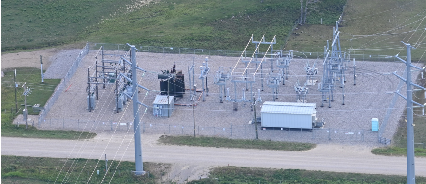
The existing Lacombe Substation.
