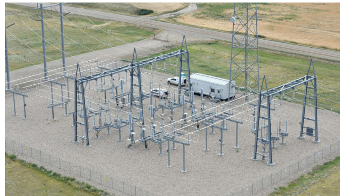
Left photo: The new Leedale switching station will look similar to the picture to the left.
