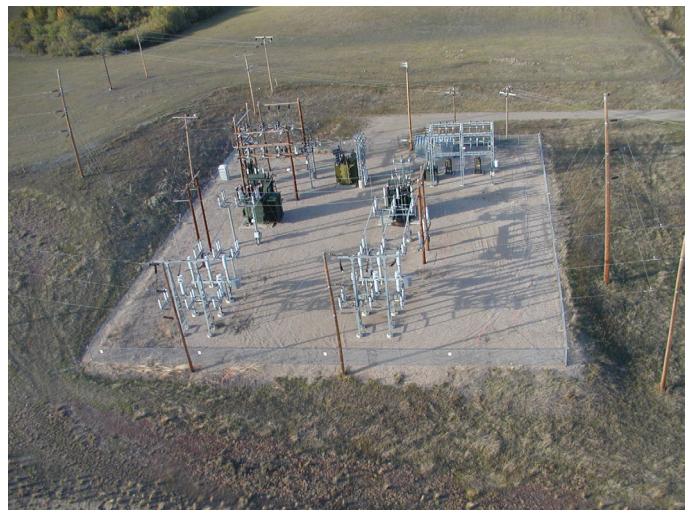
Right photo: AltaLink's existing Edgerton Substation, within which AltaLink proposes to construct a new telecommunications tower and control building.
