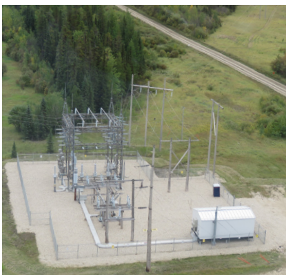
Top photo: Some of the monopole structures will look similar to the above.
