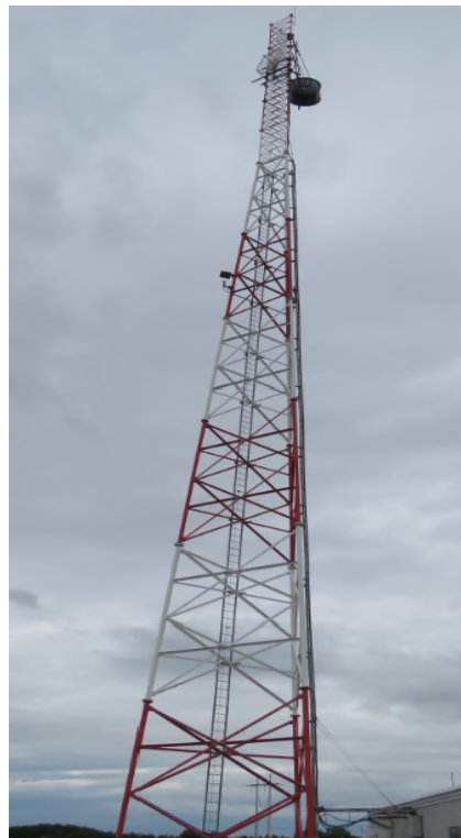
Top photo: An example of the existing structures on the 924L/927L transmission line.
