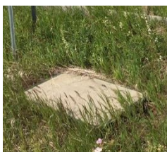
The underground conduit box will look similar to the image on the right.
