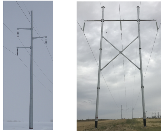
For the proposed 715BL transmission line, the monopole structures will look similar to the photo on the left, and the H-frame structures will look similar to the photo on the right.
