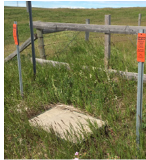
Right: The underground conduit box will look similar to the image on the right.
