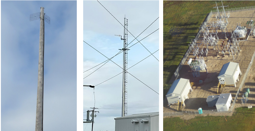
The existing telecommunications pole on the left.
